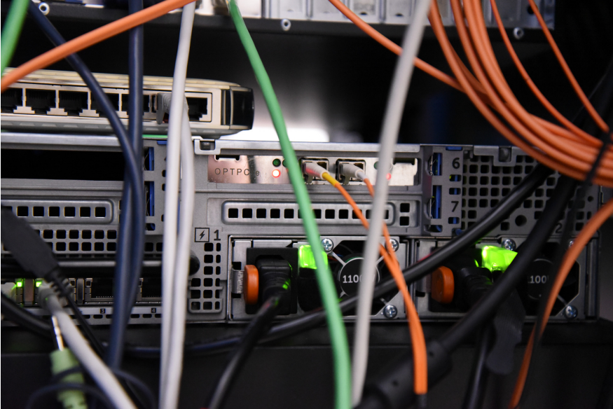
Figure 31: Example of a OPTPCI-e #015 board horizontally installed in a Dell PowerEdge R720.
