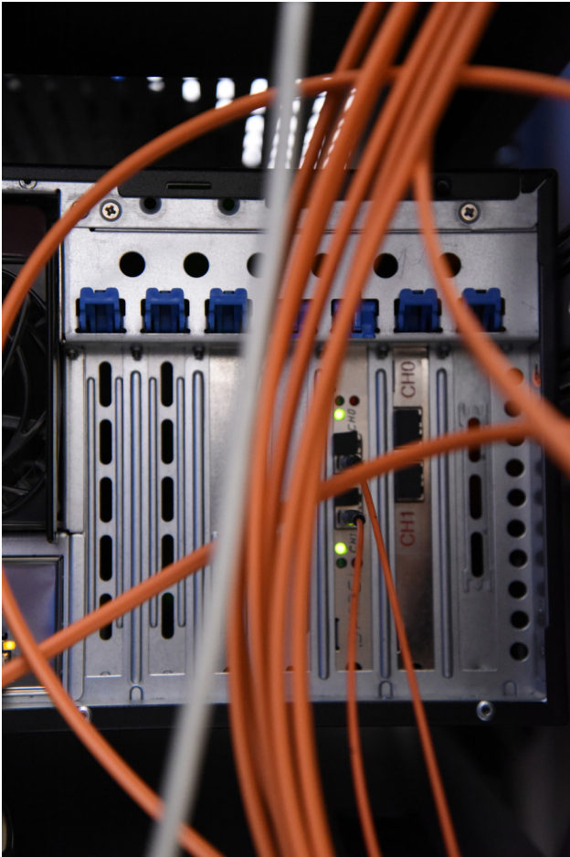
Figure 36: Example of two OPTPCI-X boards vertically installed in a Transec Workstation (2 Opteron-4C, 2382).
